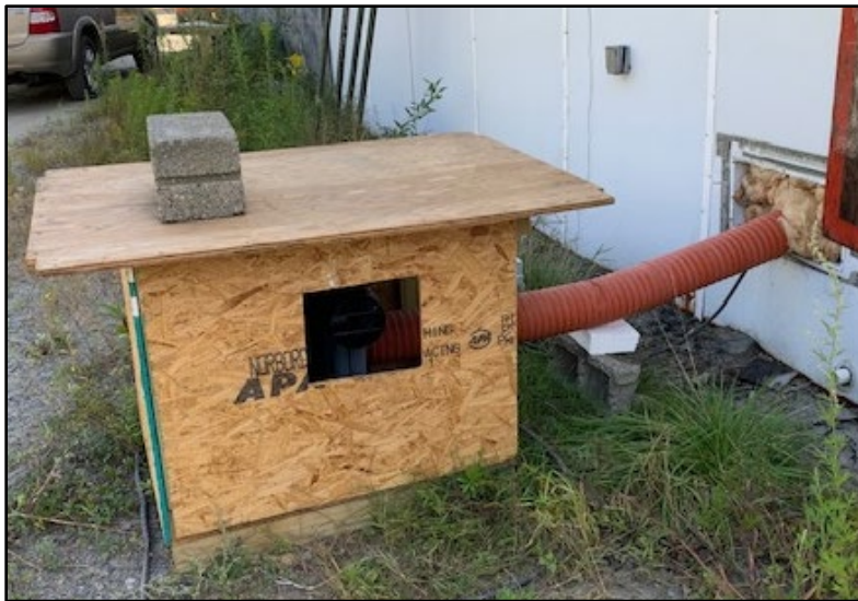
Figure 5. Exhaust fan located outside of the MEF within a wooden housing to protect against rain. A Silicone hose runs into the MEF to the test vehicle.
